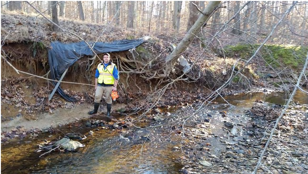
Figure 9: Stream bank incision >6 feet (vertical instability) from bed. Photo was taken downstream from sampling reach.
