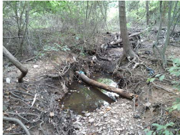
Damaged channel showing aggradation, erosion, and debris
