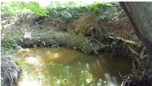
Upstream portion of reach near residences showing severe erosion
