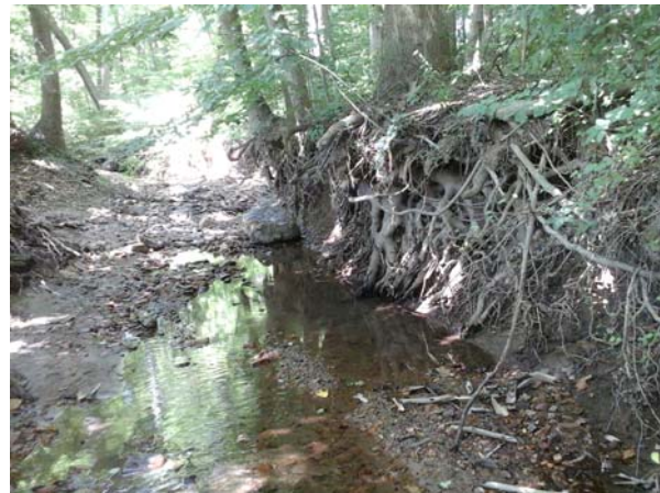
Exposed root systems in widening stream channel
