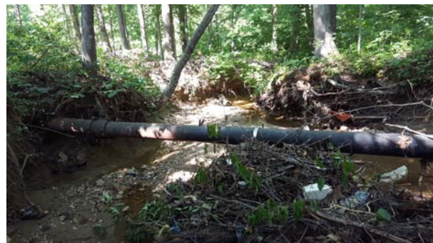
Downstream portion of reach showing exposed sanitary sewer line
