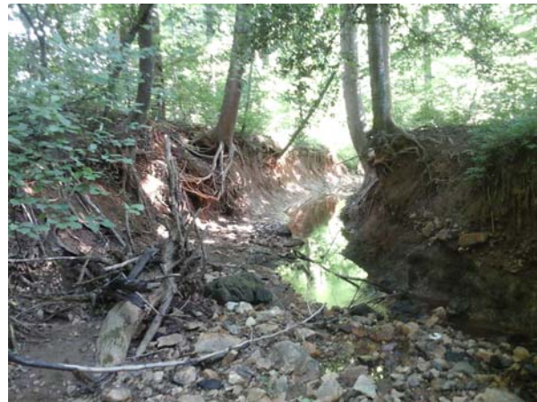
Section of stream showing damage to both banks
