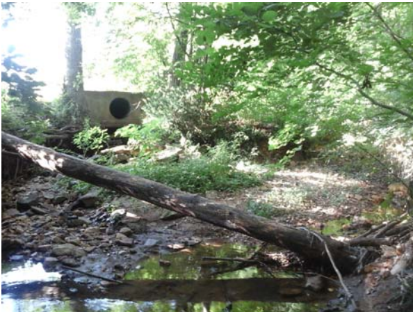
Impacted area downstream of outfall
