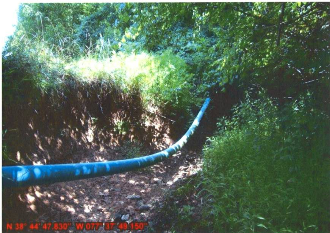
Photo 2: Exposed irrigation piping is common along the stream channel
