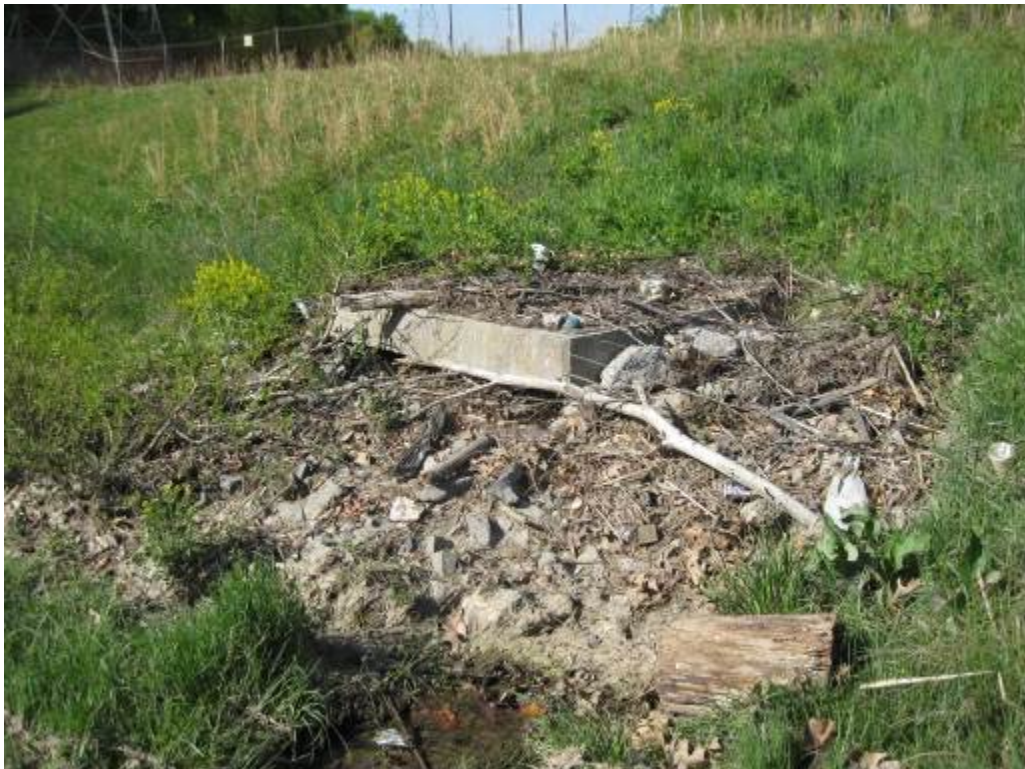
2. Facility 19. Existing riser is clogged with sediment and debris.
