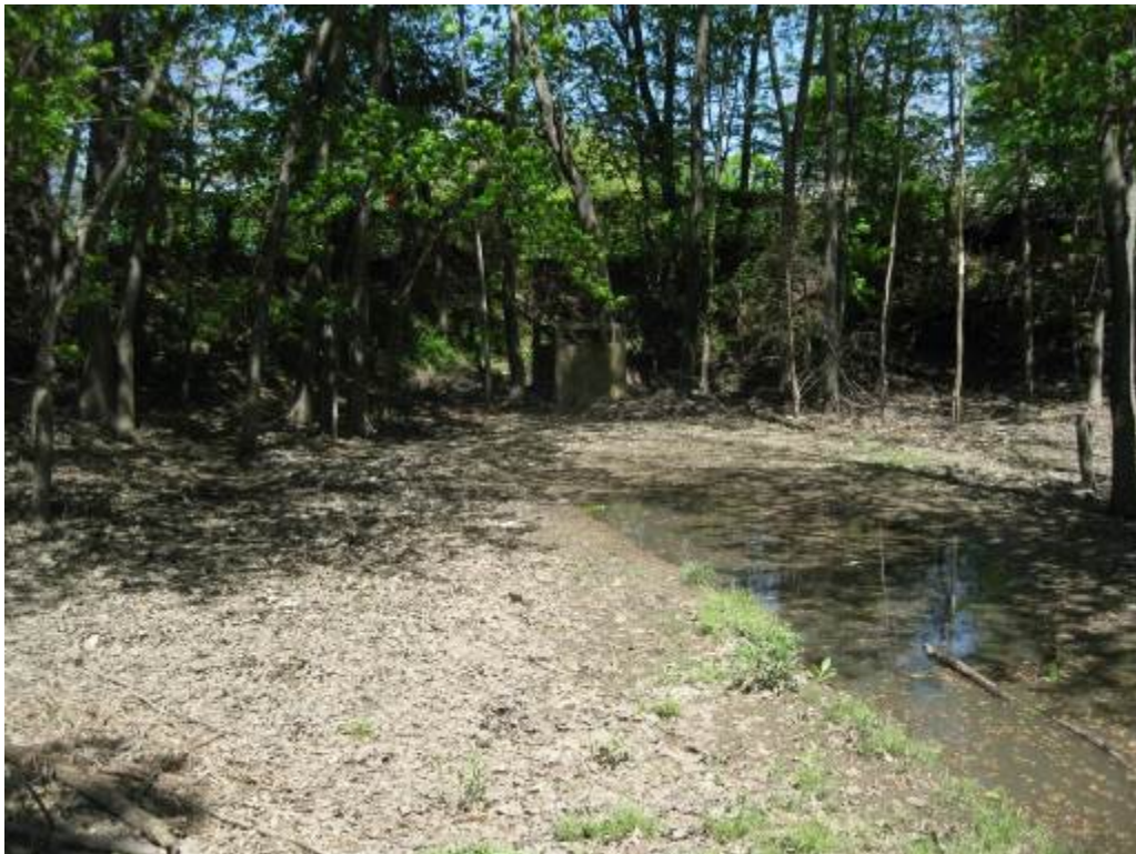
26. Facility 9026. Looking at riser in background with stagnant water in upstream channel and ponding area.
