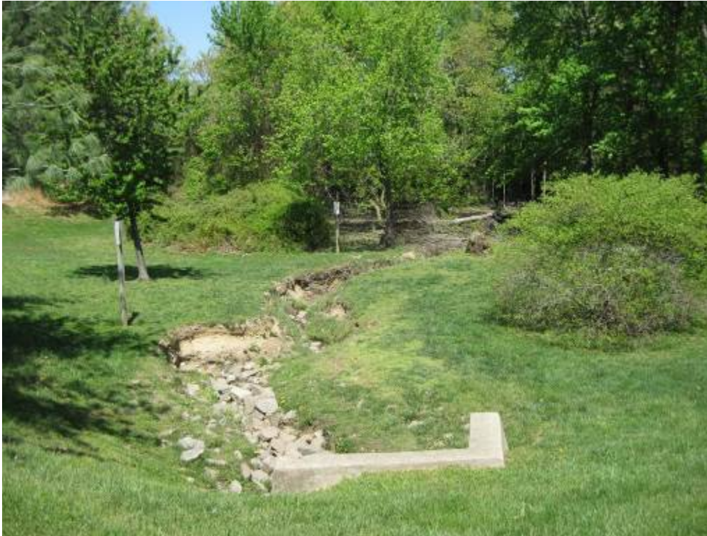
29. Facility 9026. Looking downstream at eroding channel that drains into the facility.
