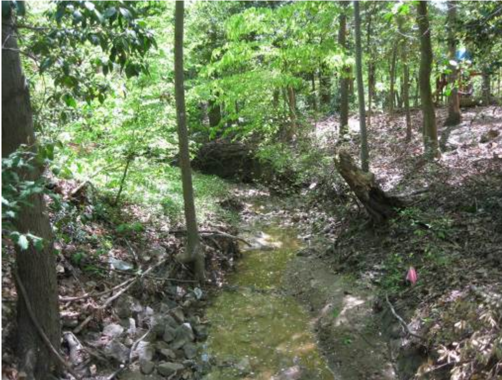
53. Facility 465. Looking downstream at incised channel showing active signs of erosion. Notice proximity of adjacent residences.
