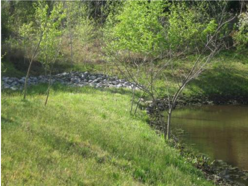
47. Facility 454. Looking at riprap along emergency spillway and small trees on dam.
