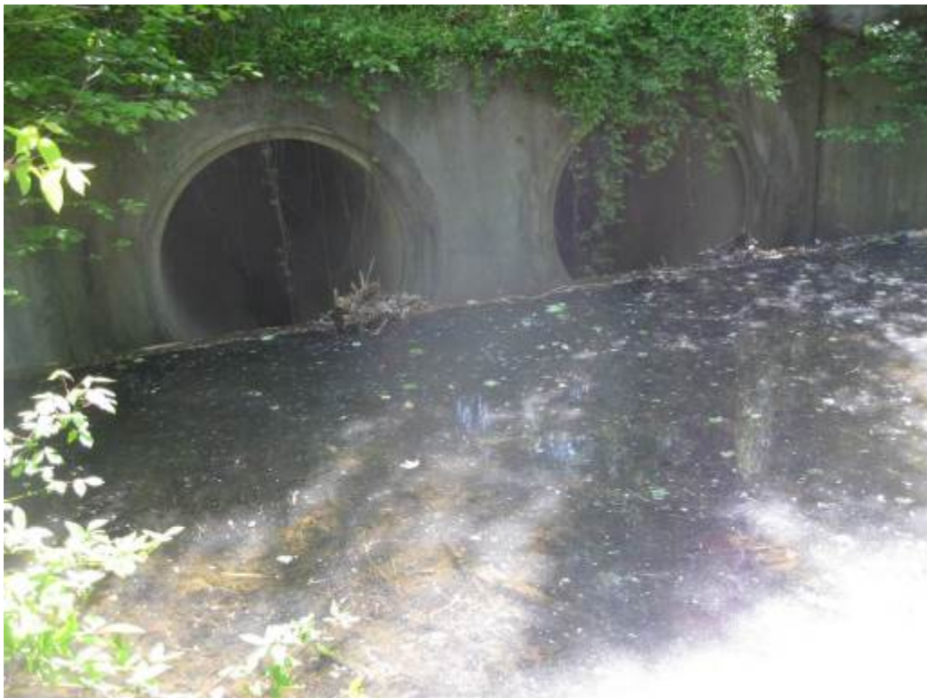
38. Facility 201. Weir wall upstream of two large concrete pipes under Abner Avenue. Sediment accumulation is evident upstream of facility.
