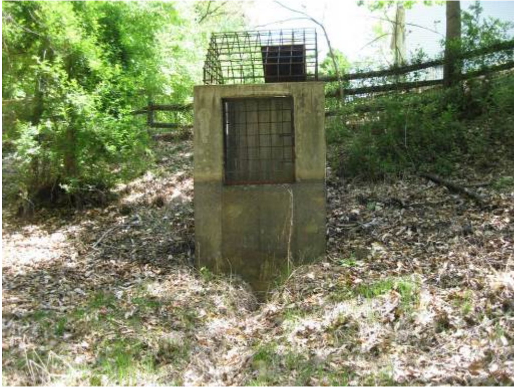
17. Facility 481. Looking at square concrete riser with angled trash rack. Wood perimeter fence is shown background.
