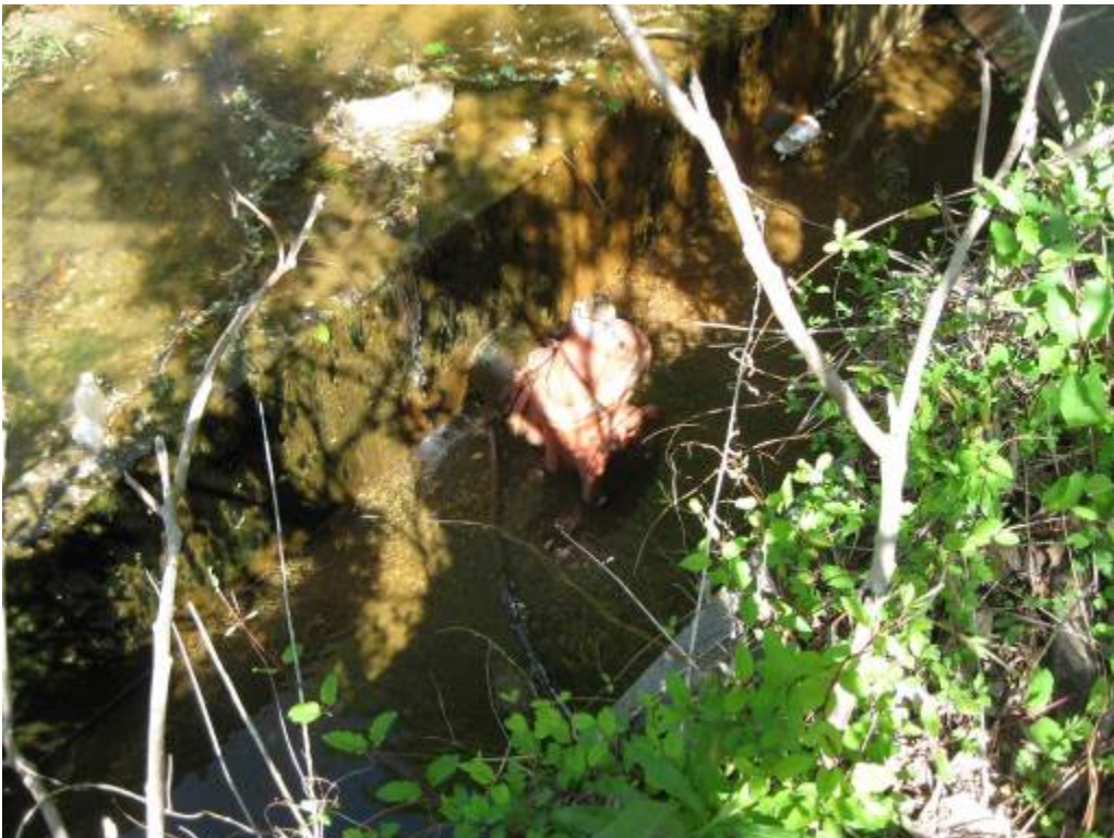
42. Facility 200. Looking at maintenance valve in weir wall. Water was draining over weir wall and through low flow orifice (approx. 2" diameter pipe through wall).
