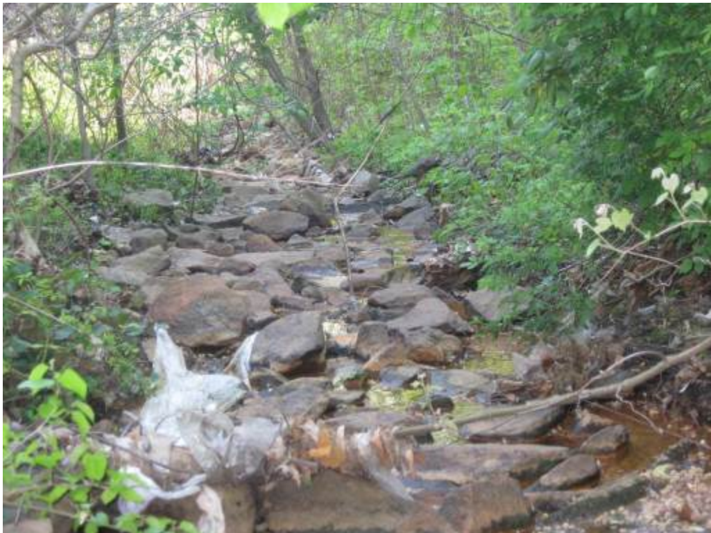
48. Facility 454. Receiving channel immediately downstream of the facility is stable with naturalized large rock.
