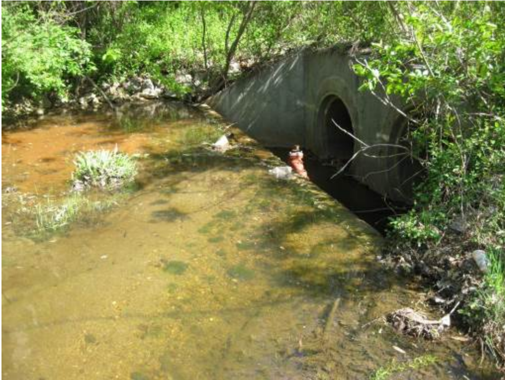
41. Facility 200. Looking downstream at weir wall and double round culverts. Sediment accumulation is evident upstream of facility.
