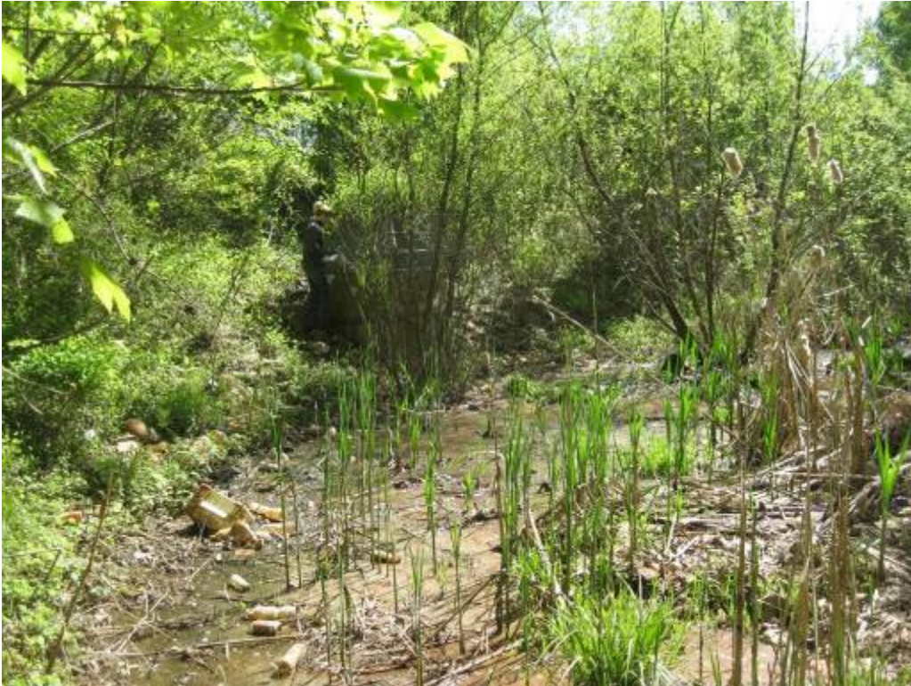
33. Facility 163. Looking at riser and ponding area. Ponding area is full of litter and fine sediment.
