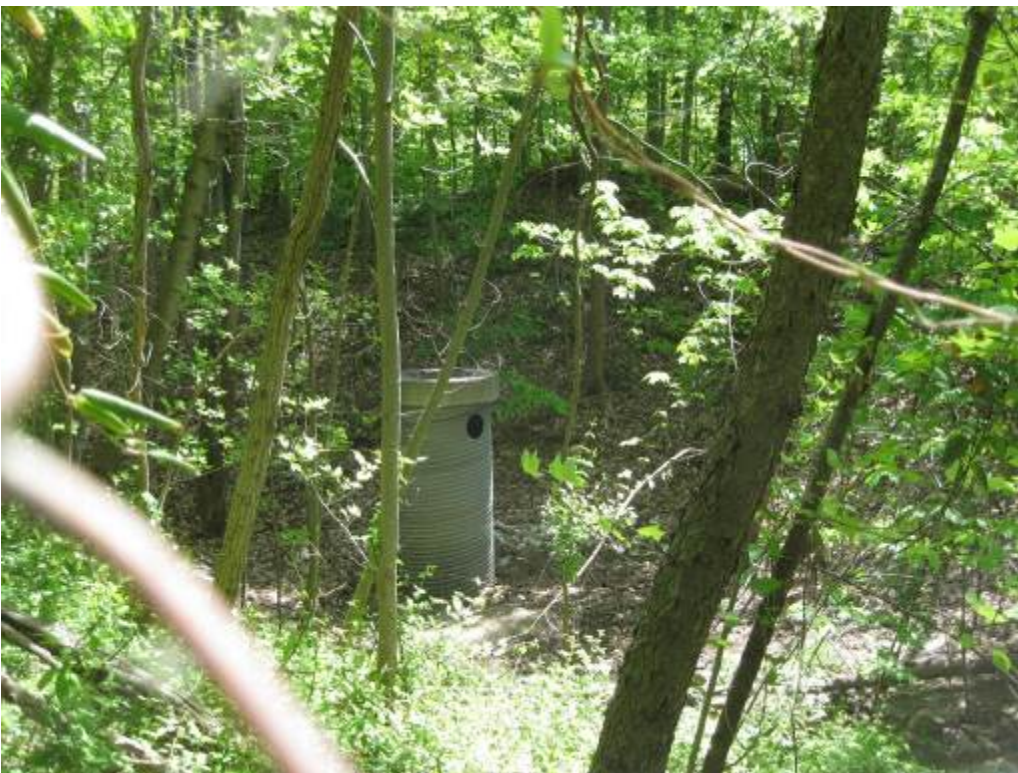
22. Facility 5147. Looking at perforated corrugated metal pipe with flat grate trash rack on top. Concrete trickle ditch runs through bottom of facility and drains into yard inlet at base of riser.
