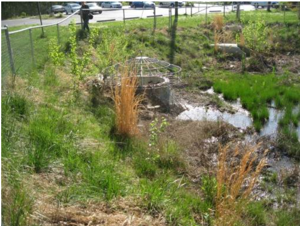
56. Facility 694. Looking at riser with anti-vortex plate and BMP orifice protected by a trash rack. Facility treats church parking lot behind the facility.
