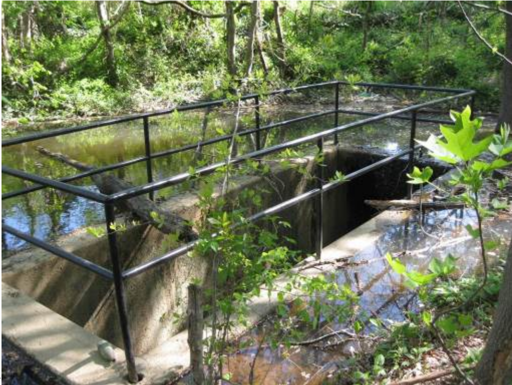
31. Facility 92. Looking at weir outlet structure. Water was overtopping weir.
