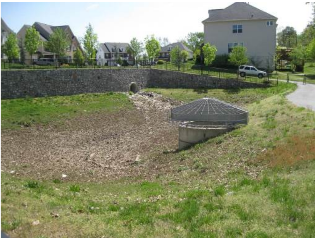
54. Facility 691. Looking at riser with anti-vortex plate and BMP orifice with extended trash rack.
