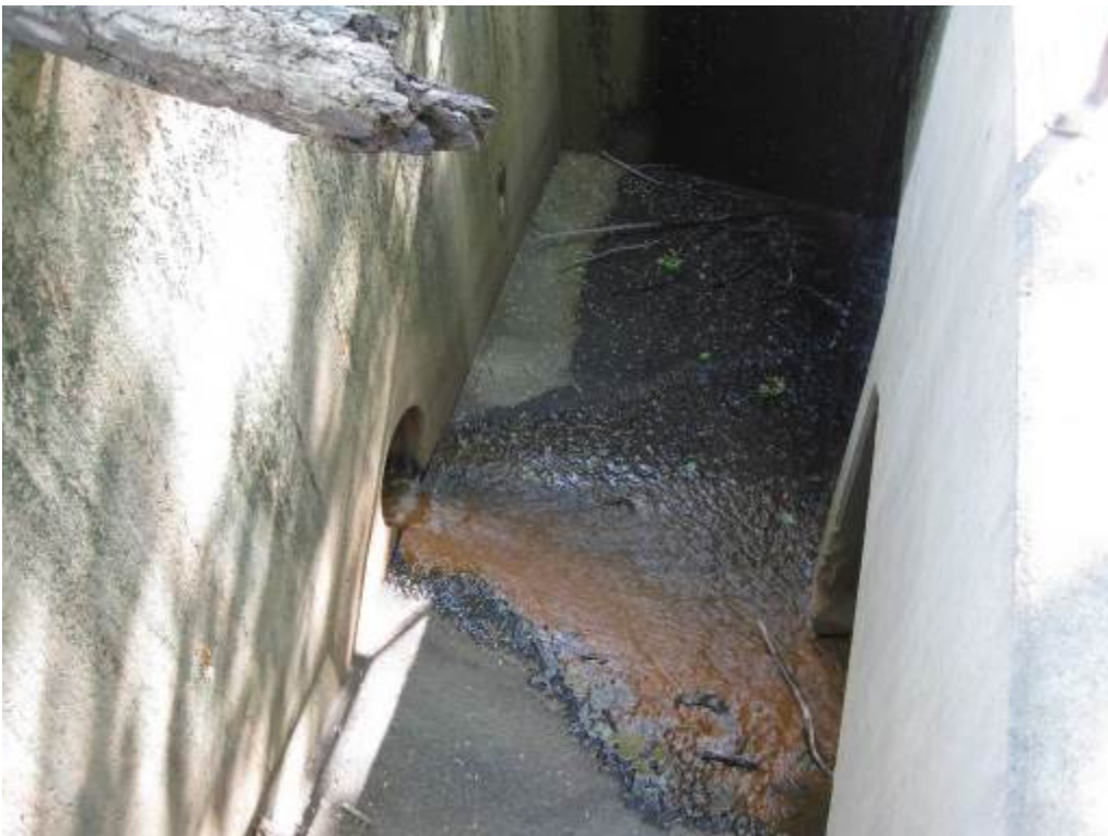
32. Facility 92. Looking at outlet which is draining to double box culvert under Interstate I-95.
