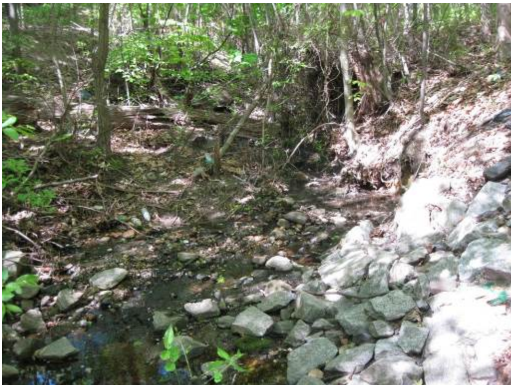
36. Facility 163. Looking at upstream channel. The channel shows some incision and bank instability.
