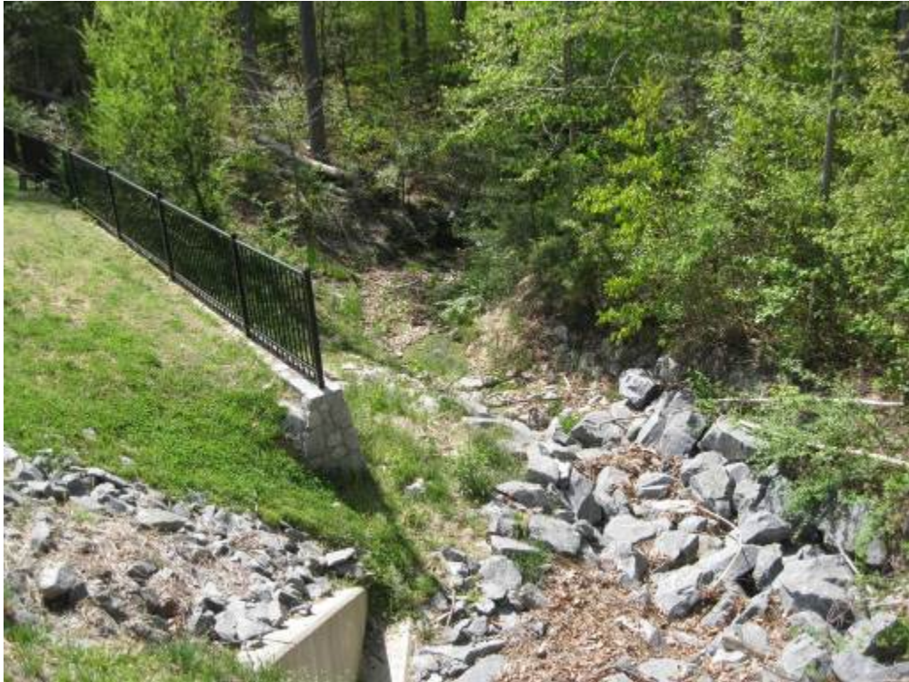
55. Facility 691. Looking at emergency spillway as it ties into stable, existing channel.
